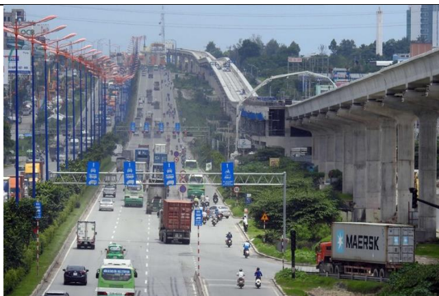
Fig 39: HCMC metro line 1 is under construction again and the government expects to launch it in 2021
